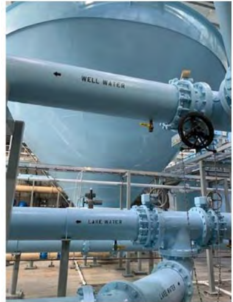
New Taylorville Water Treatment Plant
