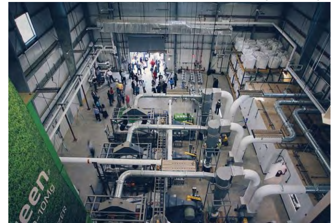
MWRD/Ostara Nutrient Recovery Facility
